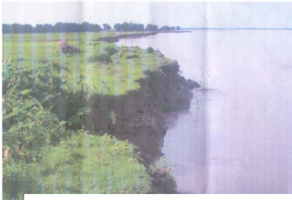
Photograph-4: Erosion on Right Bank U/S of Mahananda Bridge
