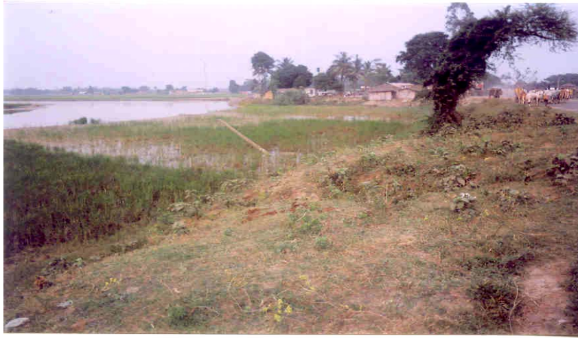
Photograph-6: Erosion on Left Bank of Bagmati River Damaging the Habitats on Outer Bank of 90° Bend U/S of Bagmati Bridge
