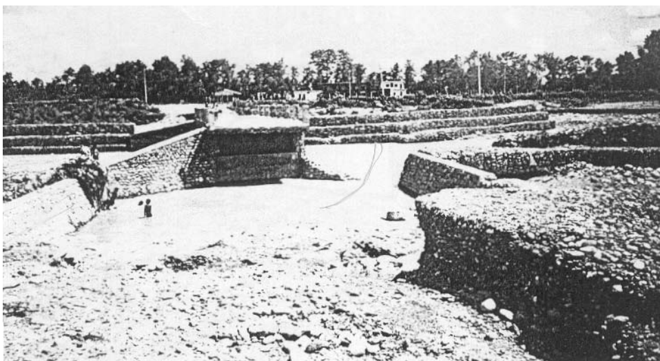
Photograph-1: Outflanking of a vented causeway on the stream 'Danab Khola' in Nepal
